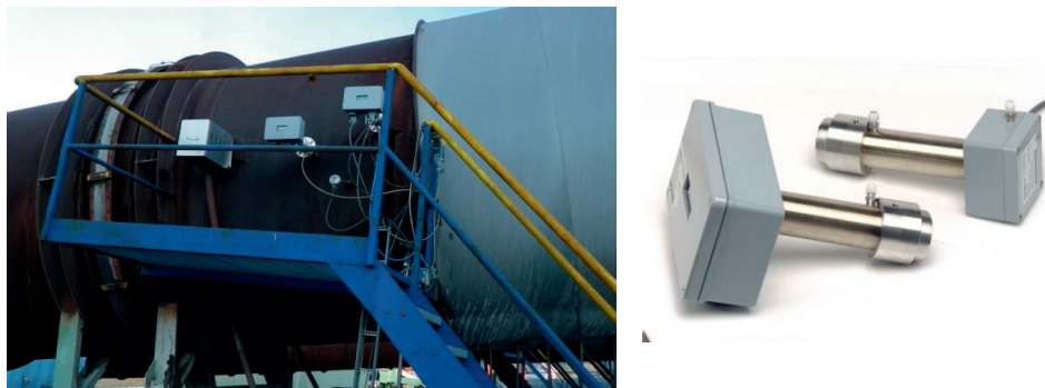
Figure 6.8: Industrial setup for NO measurements at the plant
