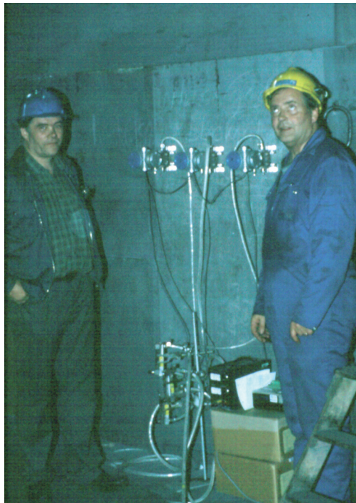
Figure 2.7: Installed differential pressure cells for measuring the furnace crater pressure in a ferrosilicon furnace and the operators while setting up the connections.
