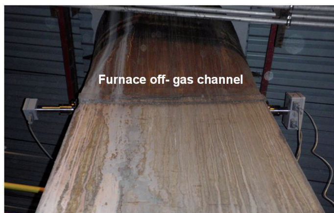
Figure 6.38: The NEO LaserDust MP system installed on the off-gas channel of a silicon producing furnace at Elkem Salten plant. The industrial tests have been performed in April 2010 (Grådahl [2010]).
