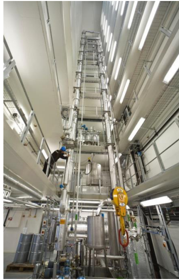
Figure 4. Tiller research pilot plant at SINTEF and main specifications.
