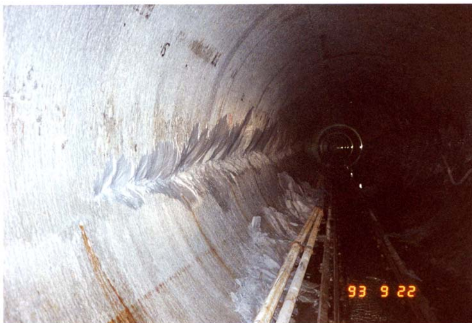
Figure 2.8 'Dog-earing' problem caused by overstressing (photo by Broch, 1993).
