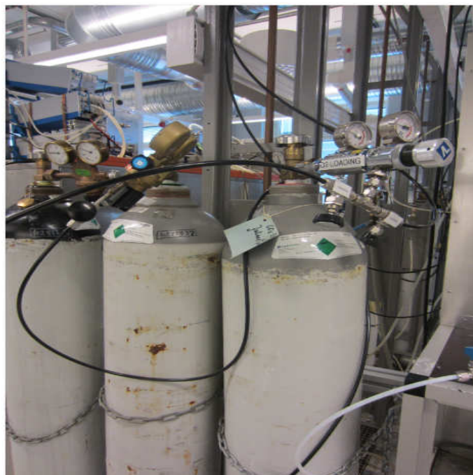
Figure 3.7 CO 2 cylinders for CO 2 loading system
