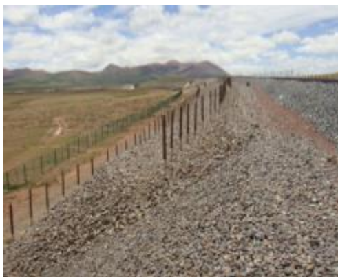
Figure 3-6: Thermosyphons at railway embankment (Yandong et al. 2013)
