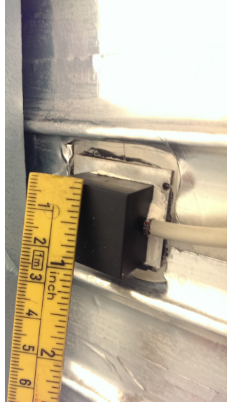
Figure 2.15: A finished sensor glued to the tank wall, located between aluminium tape covered heating cables.
