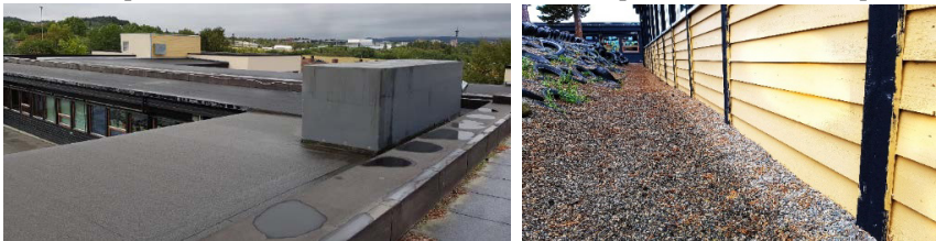
Figure 1. (left) The casings for ventilation ducts and technical pipes. (right) The clogged ventilation aperture of the wooden cladding in parts of building A.
