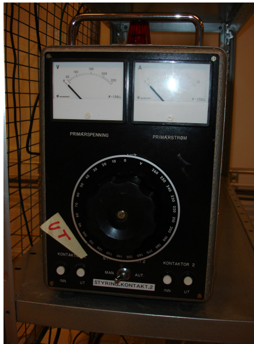
Figure 3.5: The variac used in the setup, supplying the low voltage input to the high voltage transformers.
