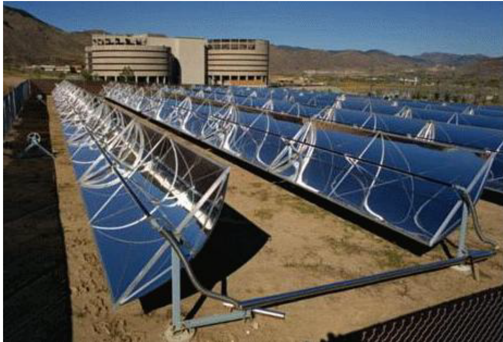
Figure 3.1: Picture showing parabolic trough concentrators at Kramer Junction. Source: NREL.
