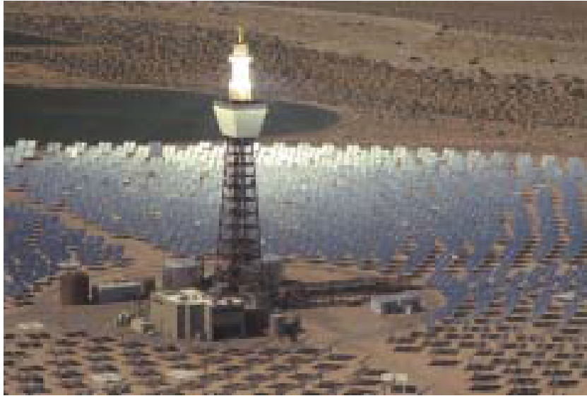
Figure 3.2: A picture of Solar Two, the prototype power tower. Some 1,926 heliostat mirrors are used to produce 10 million watts of electricity. Source: Sandia Laboratories.
