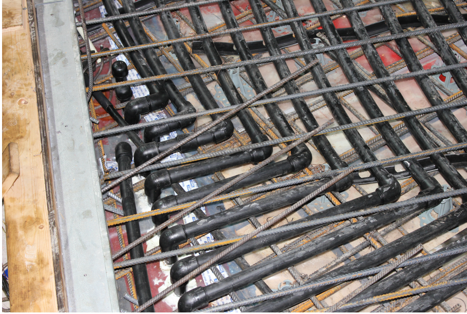
Figure 1.1: Cooling pipes in the concrete. The pipes cover the whole rink and alternate between inbound and outbound. Although the picture is from Hamar Olympic Hall, the same setup is used in Schjong Ice Rink.
