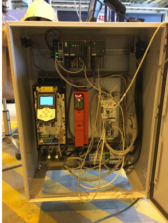
Figure 2.3: Electrical cabinet to keep the electrical system separated from water
