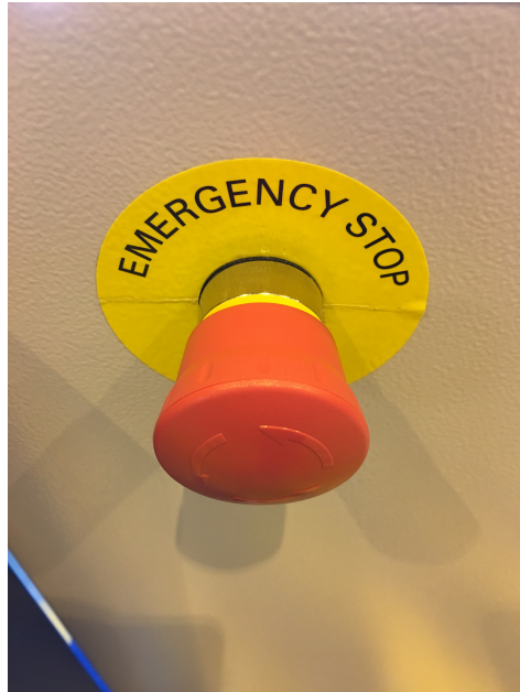
Figure 2.5: Emergency stop button attached to the electrical cabinet
