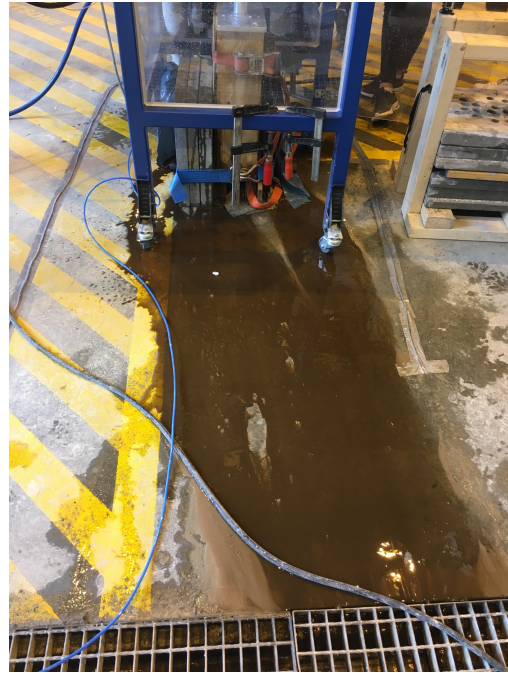
(b) Return flow from annulus indicating asphalt was being drilled
