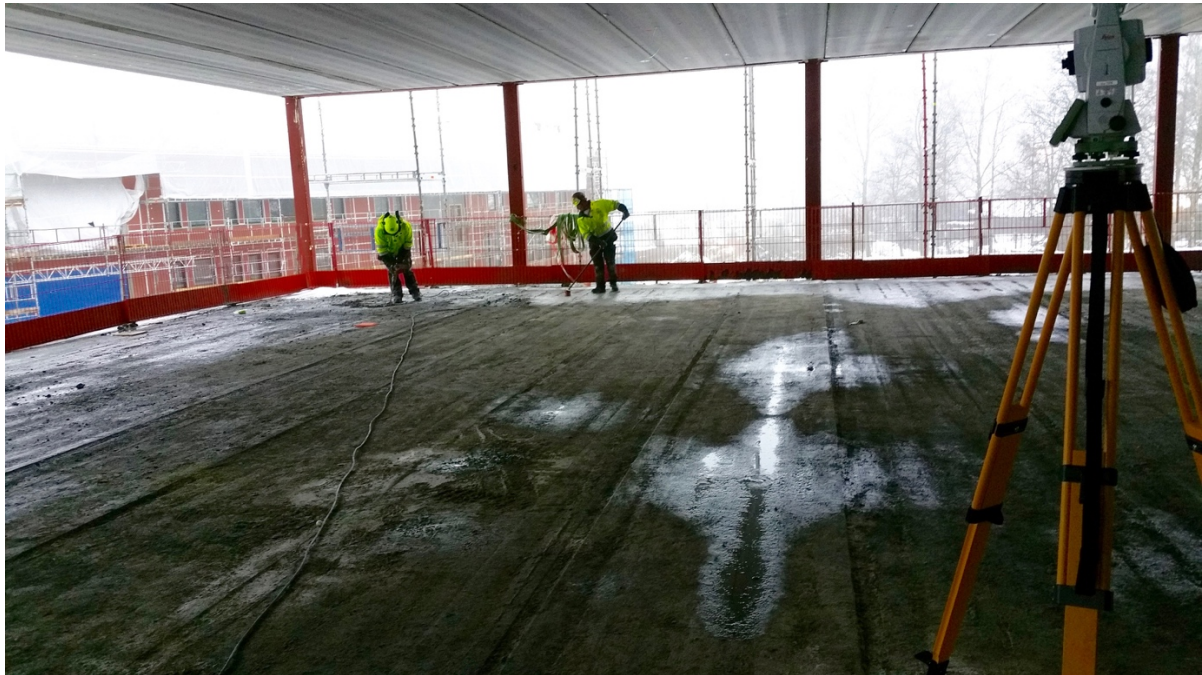
FIGURE 4.22 ELECTRICAL CHISELING WORK CAUSING POWER FAILURE (OLE ROSENLUND, 2017)
