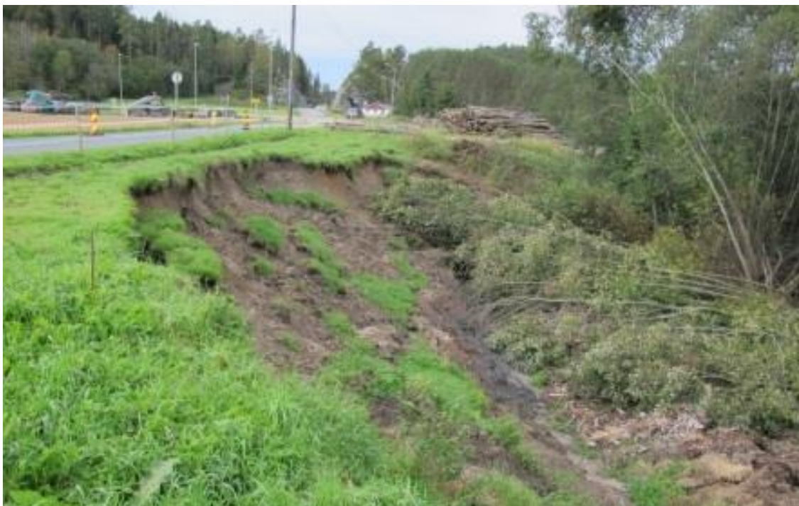
Figure 3. Soil slip caused by a weak layer, Åby in Telemark county, Norway(Håland, 2012)
