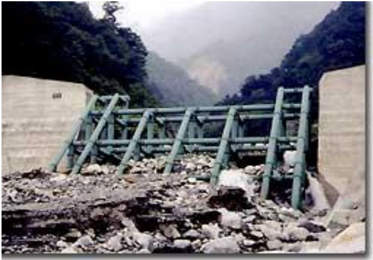
Figure 10. Open steel pipe in sabo dam ( http://www.ktr.mlit.go.jp/fujikawa/english/project/ )
