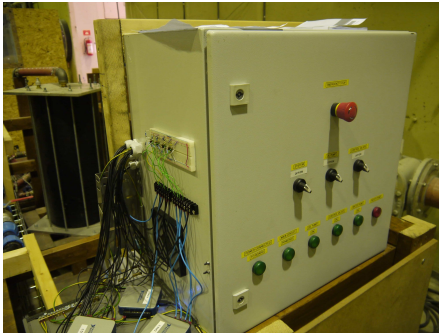
(a) Control cabinet
