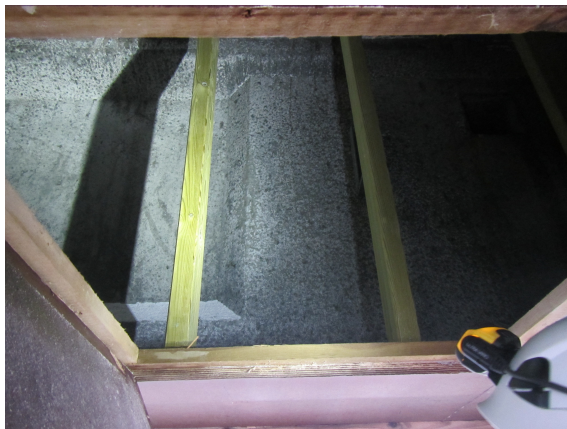
Figure 4.4: Efflorescence on the NIB-beam. Picture taken slanted upwards from the inspection hatch
