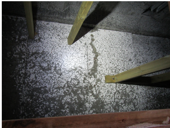
Figure 4.5: Efflorescence in the underside of the bridge deck. Picture taken vertically upwards from the inspection hatch
