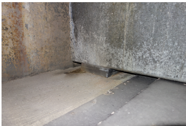
Figure 9.1: Image from the excursion showing the rubber bearing at the beam end
