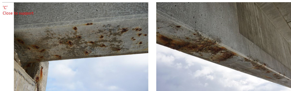
Figure 11.7: Close-ups of corrosion area 'C' near the east abutment
