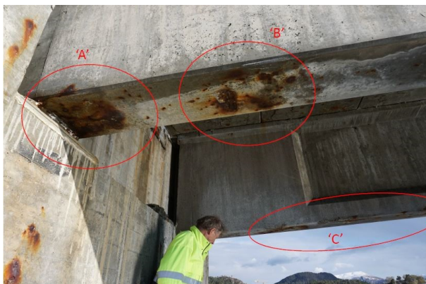
Figure 11.6: Corrosion near the east abutment
