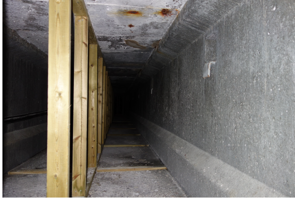
Figure 11.4: Efflorescence on the underside of the bridge deck near axis 10
