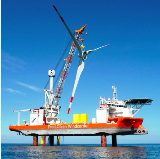
(a) Fred. Olsen Brave Tern lifts a rotor and blade assembly for installation (Fred. Olsen Windcarrier, 2016a)
