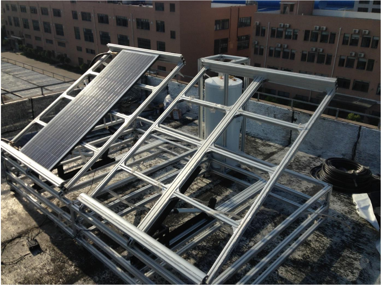
Figure 3-8: Solar test rig with one PV/T component connected to a tank
