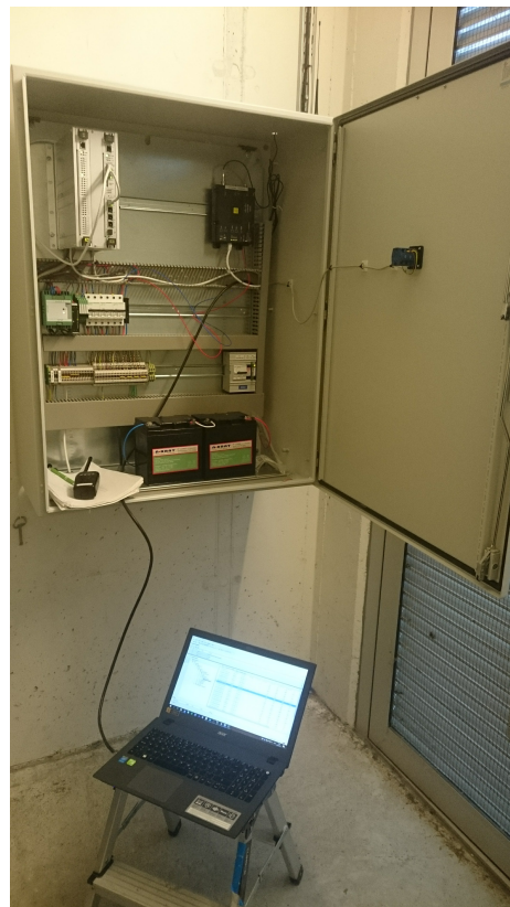
Figure E.7: Connection to grid protection through RTU in DG1.
