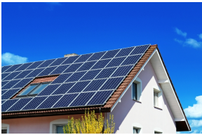
(a) Roof mounted photovoltaic panels.
