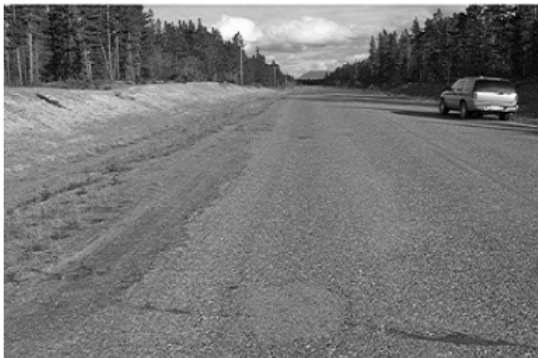
(a) Cracked pavement due to frost heave in a city street in Yukon, Canada (from Dore and Zubeck (2008))
