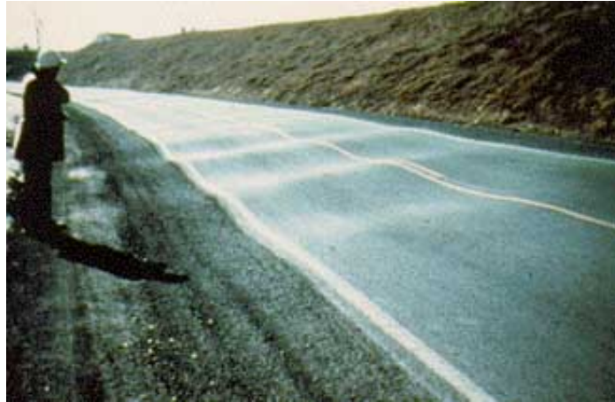
Figure 1.5: Frost heave damaged a road (from DiMillio (1999))
