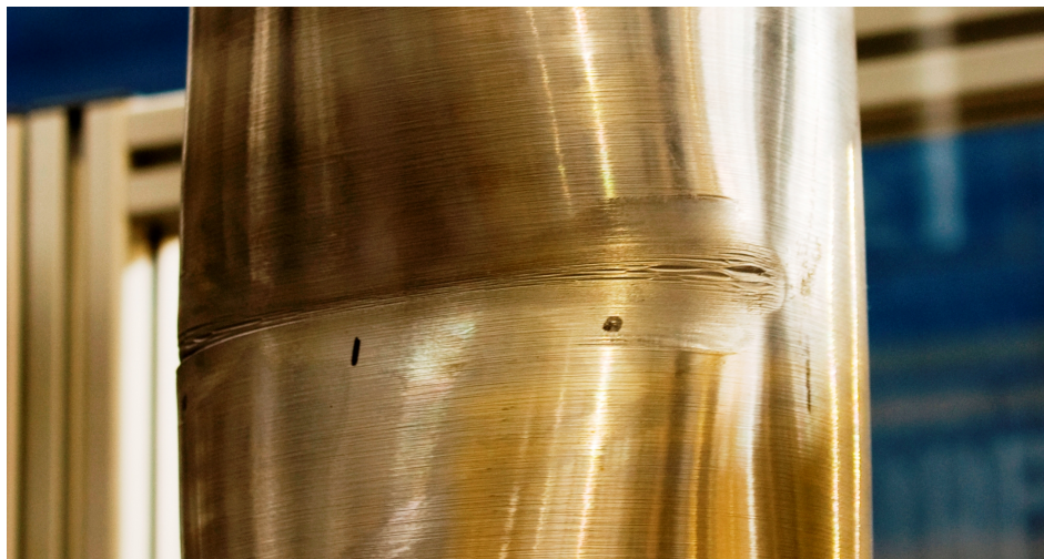
(c) Surface cracks in pipe A
