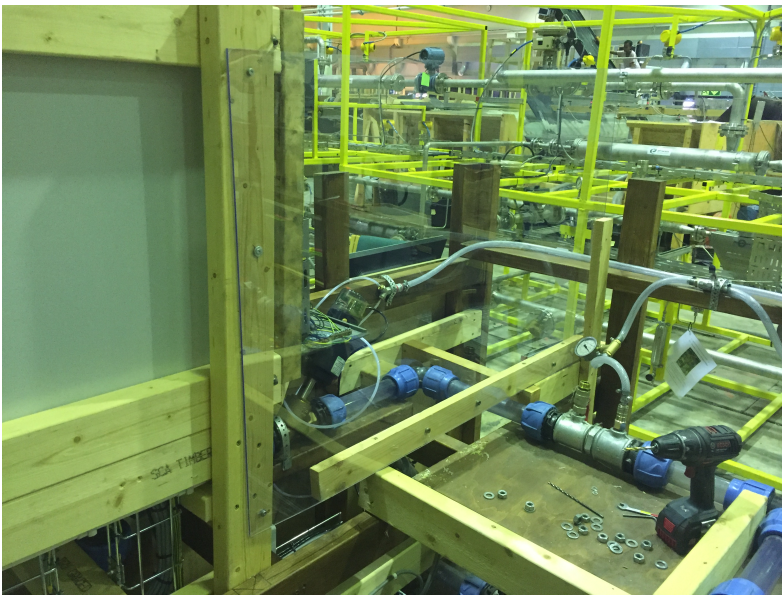
Figure 3.28: Control station protection
