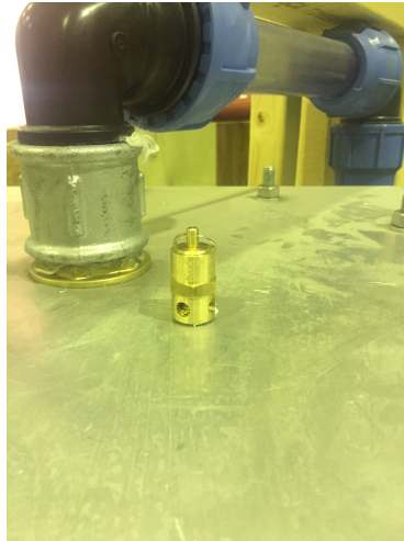
Figure 3.26: Pressure release valve (PSV)
