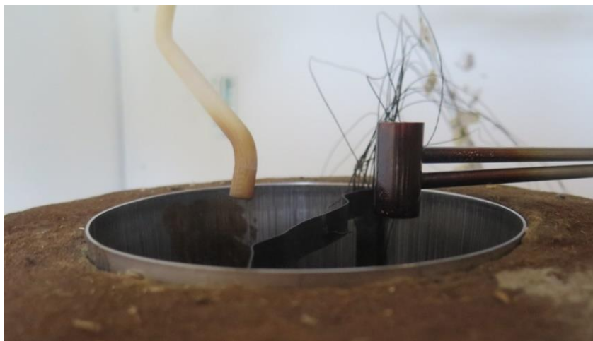
Figure 26: Close-up picture of the gas measurement unit and bidirectional probe position with regards to the pipe.
