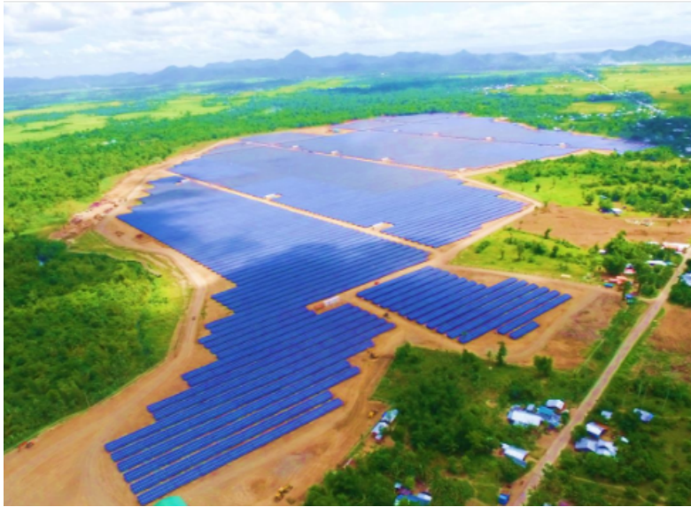
Figure 2.2: Sepalco 50 MW PV farm. Source: Sepalco
