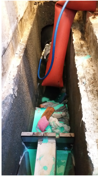
Figure 4.6: Silicone and hardening leaking from the framework [Photo PPN]
