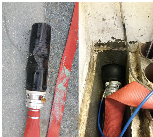
Figure 4.2: Left: The pipe plug with hose to redirect the flow. Right: The pipe plug in operation [Photo PPN]
