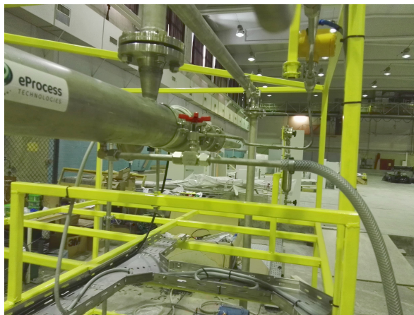
Figure 5.1: Workshop water feeding system connected to the CSL.
