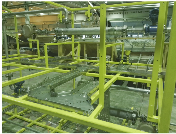
Figure 3.13: Example of cable trays for Skid 2.
