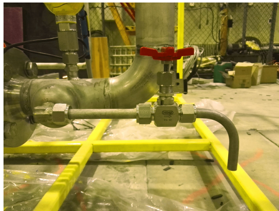
Figure 3.5: Example low drainage point in the CSL.
