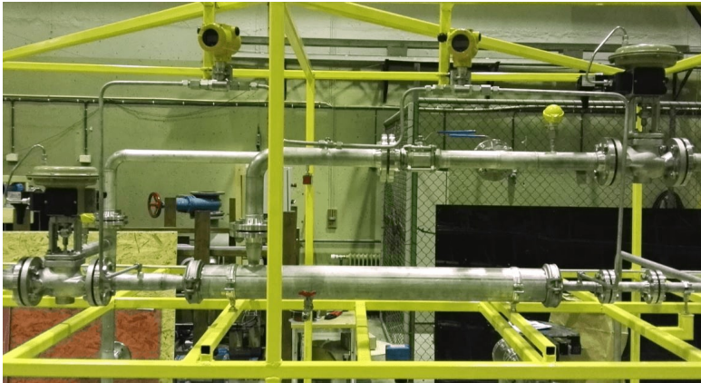
Figure 3.8: Example of installed PDT on the third vessel housing.
