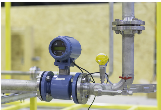
Figure 3.6: Installed electromagnetic flow meter with black wiring for process grounding.
