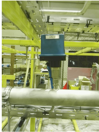
Figure 3.11: Installed pressure switch in the CSL.
