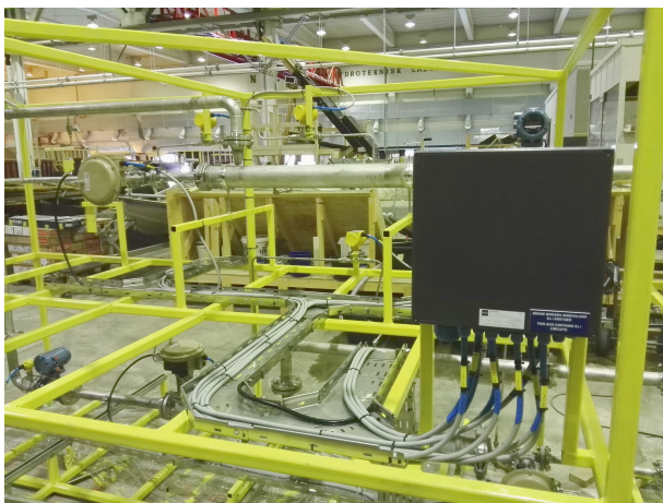
Figure 3.16: Cabling and installed IS junction box on Skid 1.
