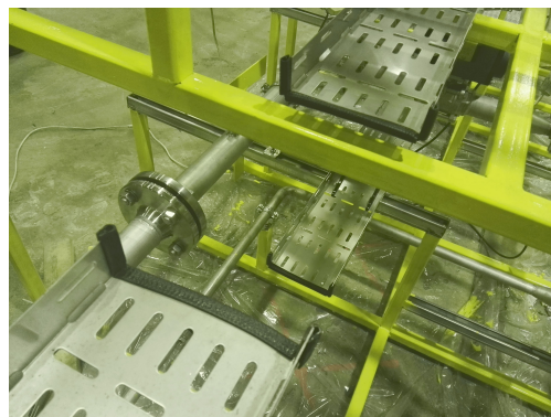
Figure 3.14: Protective lists on cable trays between Skid 1 and Skid 2.
