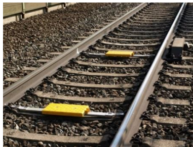
Figure 2.5 Eurbalise (Balise) in between railway track
