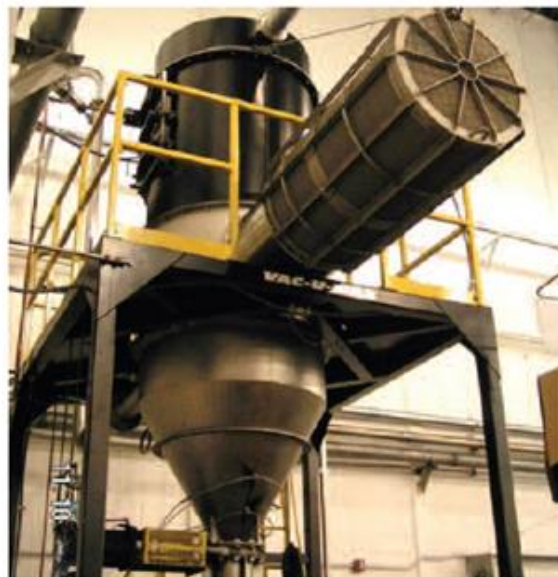
c. High-speed isolation valve on system's tubing leading to dust collector
