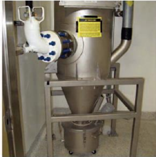
b. Flame-arresting vent on system's dust collector
