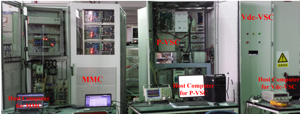
Figure 1.6: Experimental setup of VSC- and MMC-HVDC system.
