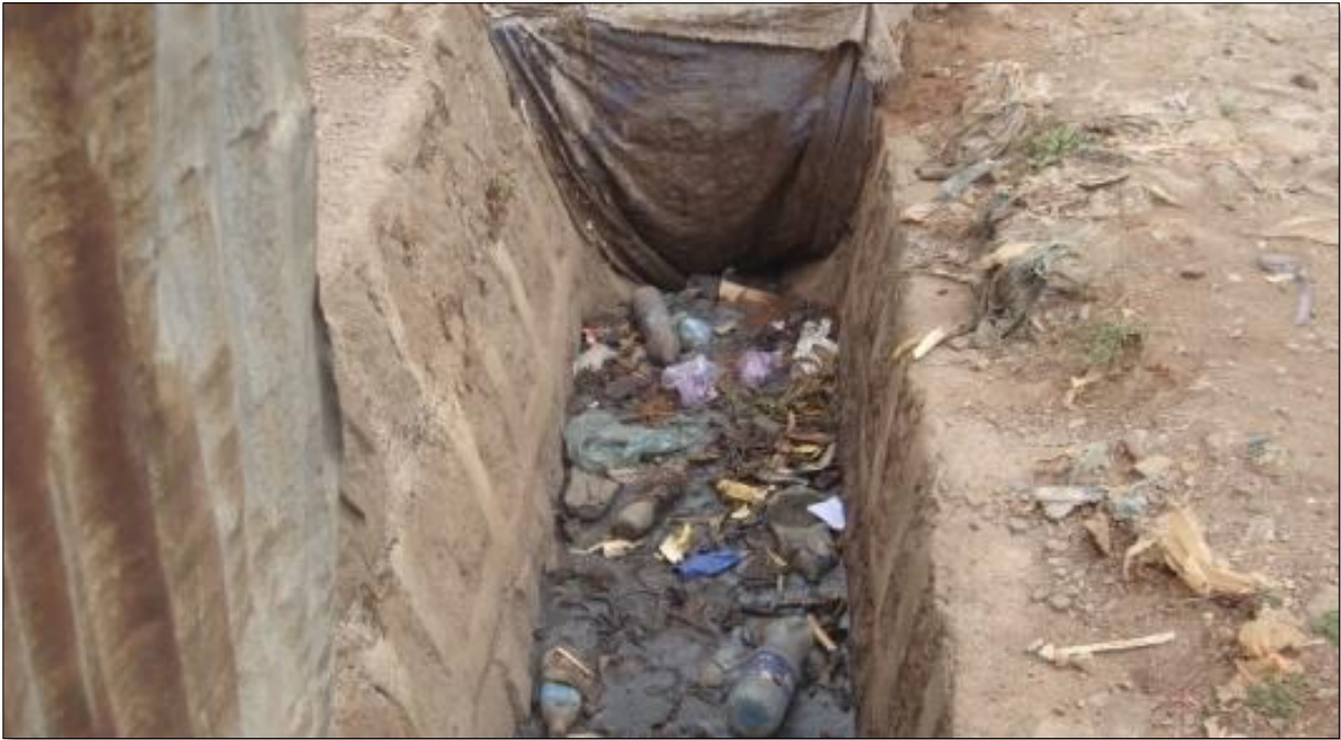
Figure 5.8: Improper use and maintenance of drainage system
