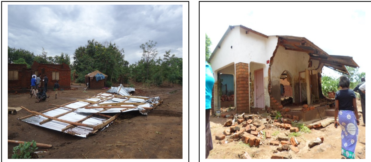
(a): House damaged by stormy wind
