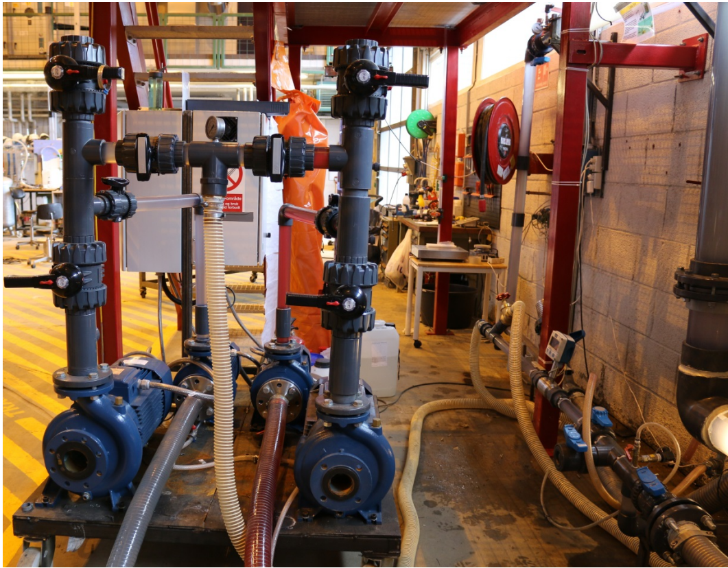
Figure 4.6: Pump manifold and connection to the displacement rig
