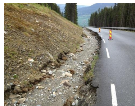
Figure 26: Erosion along the road at damage point 1-3
