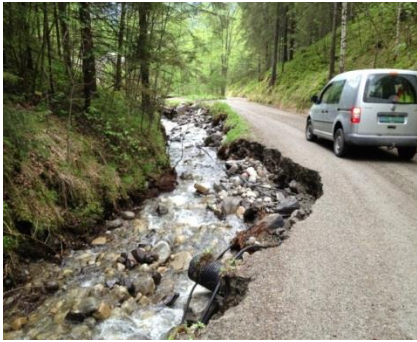
Figure 29: Damage point 8 (Foto: JBV v/Steinar Myrabø)
