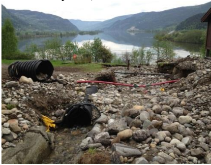
Figure 32: Damage point 5 (Foto: JBV v/Steinar Myrabø)
