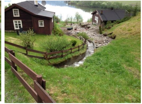
Figure 31: Damage point 5 (Foto: JBV v/Steinar Myrabø)
