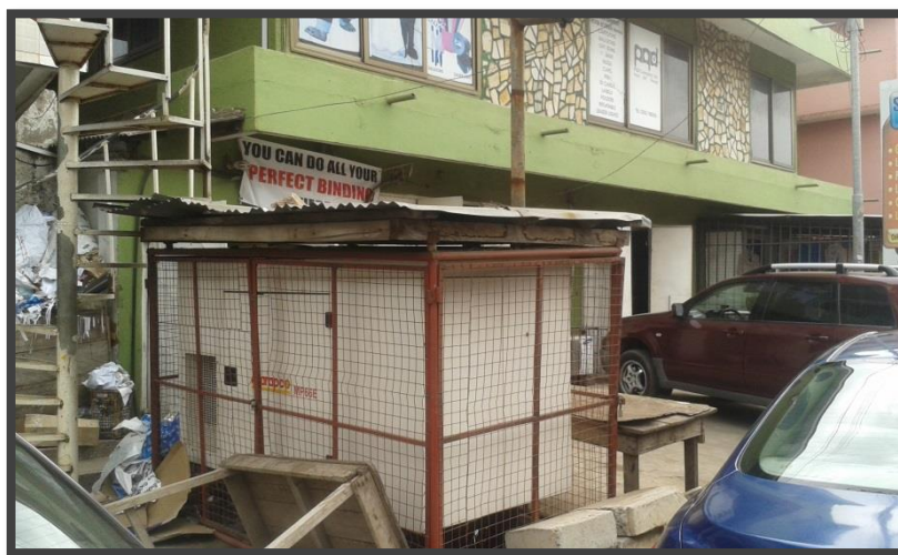
Picture 4: A standby generator for a printing press in Accra Newtown
