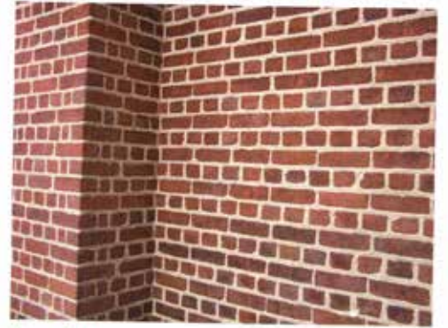
Figure 2-11 Alternating courses of brick that are laid in the stretcher position and the header position creates an English bond pattern.
