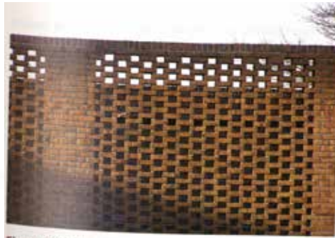
Figure 2-9 This screen wall, a modification of the Flemish bond pattern omitting the headers, encloses a building's cooling and ventilation equipment. Screen walls can be built either as a single-wythe or a double-wythe wall.
