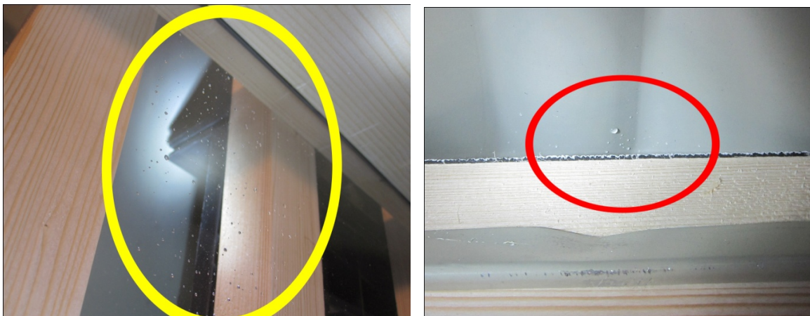
Fig. 7: The droplets of water occurring on the wind barrier, marked with a large yellow ellipse (left), and the water droplets occurring between steel fitting and steel plate roofing, marked with small red ellipse (right).
