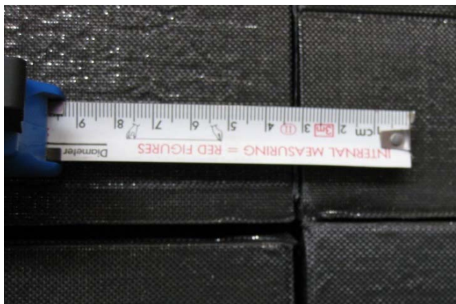
Figure 7. Irregularities in the VIP dimensions result in gaps of varying width between panels.
