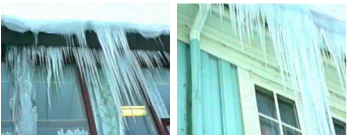
Figure 4. Large icicles in front of the glass facade of a school building, covering the windows and representing a hazard to the children (left) and large icicles blocking the window and representing a hazard to the people below (right). (Photo: SINTEF Building and Infrastructure).
