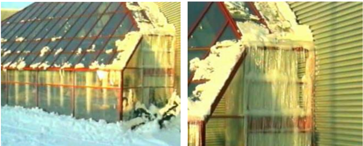
Figure 3. Large icicles covering the glass facade at a shopping centre (left) and close-up of the right part of the left photo, where the ice is completely covering this part of the glass facade (right). (Photo: SINTEF Building and Infrastructure).
