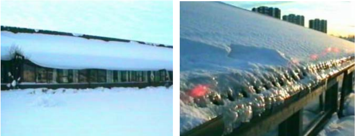
Figure 2. Snow hanging from roof and covering the glass facade of a school building (left) and rain gutter at the eaves completely full of ice (right). (Photo: SINTEF Building and Infrastructure).
