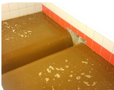
Figure 5.1.4: Overflow in filter, photo taken under backwashing.
