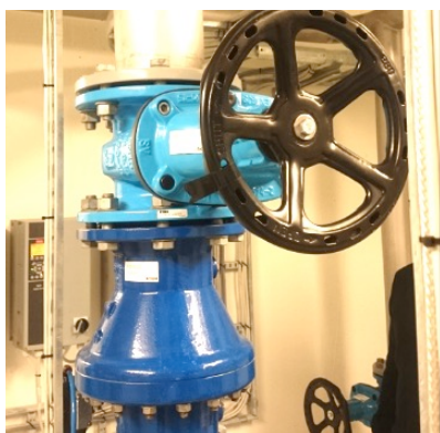
Figure 3.2.6: Gate valve above intake pumps check valve
