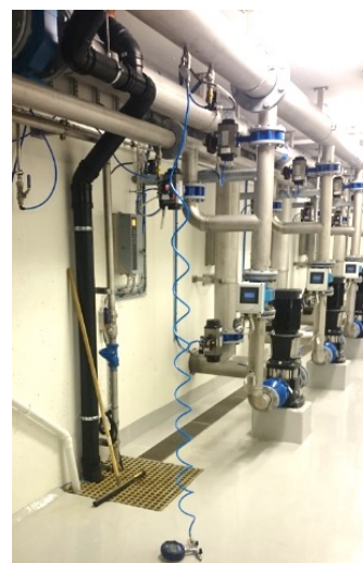
Figure 3.2.5: Pressure reading post filter pipe combination
