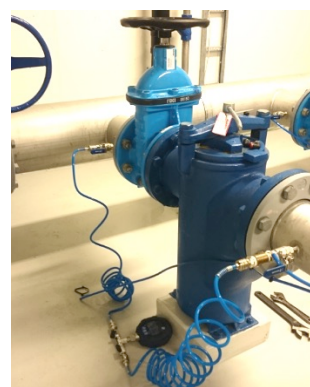
Figure 3.2.7: Pre pump filter and fully open gate valve
