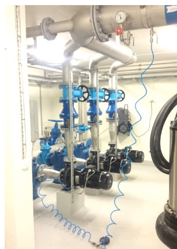
Figure 3.2.8: Pressure pre pump and post collection
