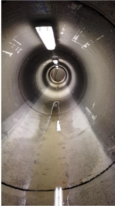
Figure 31 Detention basin (Photo: Jens H. Trandem)
