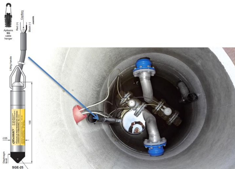
Figure 25 Left: Pressure sensor for water level measurement (aplisens). Right: Pressure sensor installed in SF2 (Photo: Jens H. Trandem).
