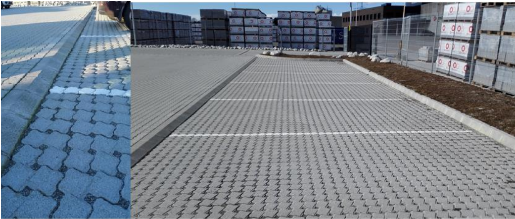
Figure 21 Transition between the impermeable parking area and permeable parking area. (Photo: Jens H. Trandem)
