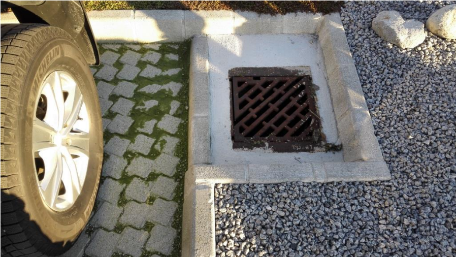
Figure 20 Design of drainage for excess water from test area 3 (Photo: Jens H. Trandem)
