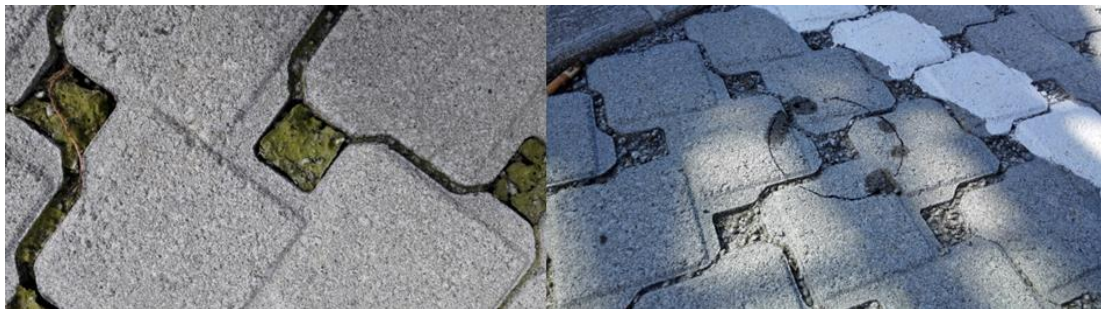
Figure 62 Picture of the joint fillings for the permeable pavement in test area 3. Lowest part to the left with green algae on top of the filling material and the upper part to the right with no algae on top of the filling material. (Photo: Jens H. Trandem)
