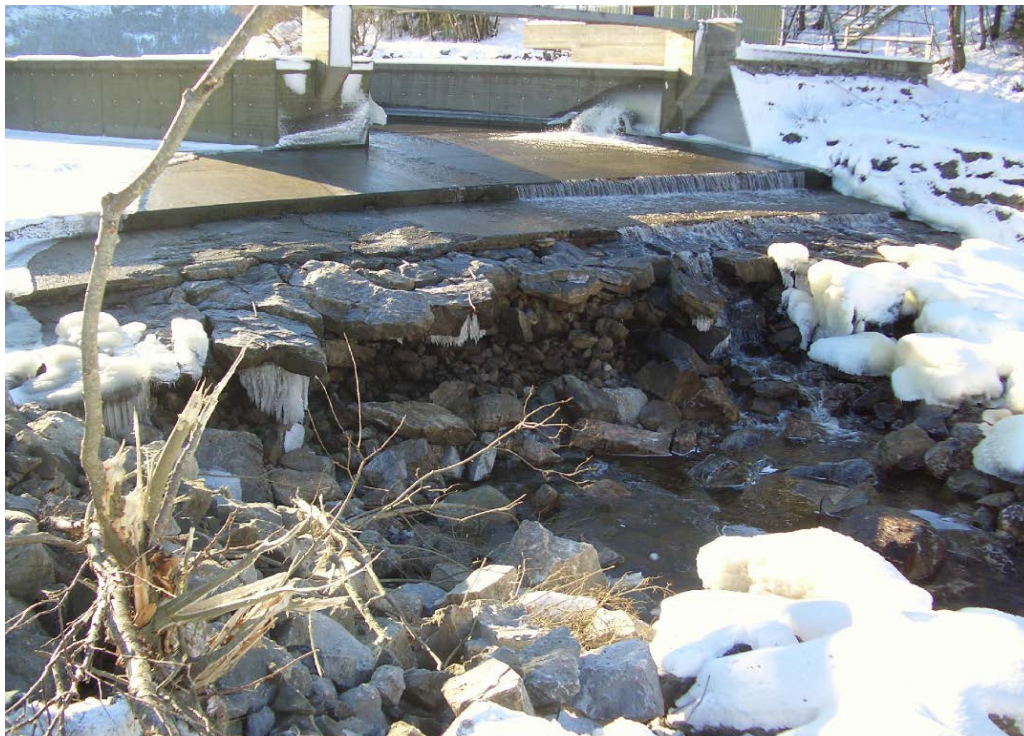
Figure 6-1: Downstream erosion during a big flood event of Lauvsnes dam Norway (Photo: Norsk Groønn Kraft)
