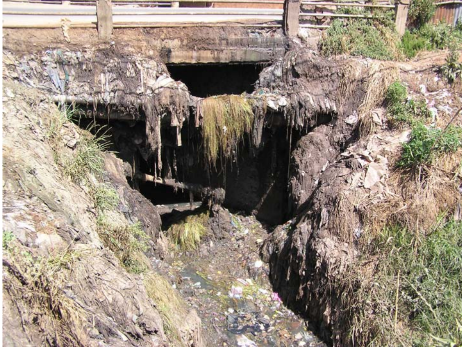
Waste in water channels.
