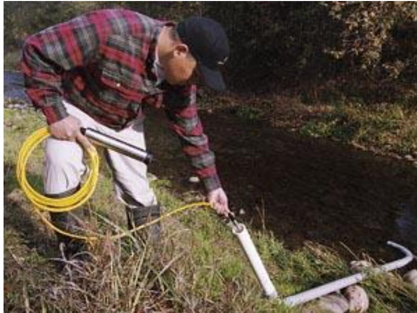
Figure 3-9. Installation example of Logger. ( www.globalw.com/products/wl16.html , 2014)
