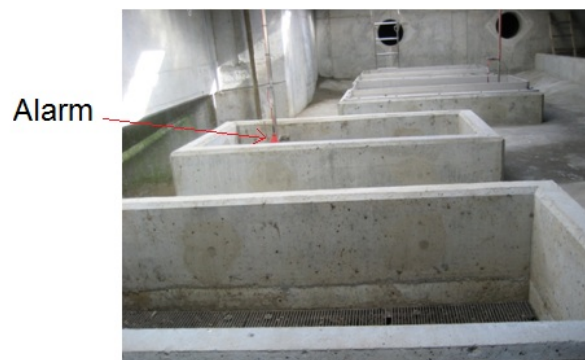
Figure 6.4: CSO overflow with alarm (Photo: Anders-Lyggard Jenssen & Lars Hem).
