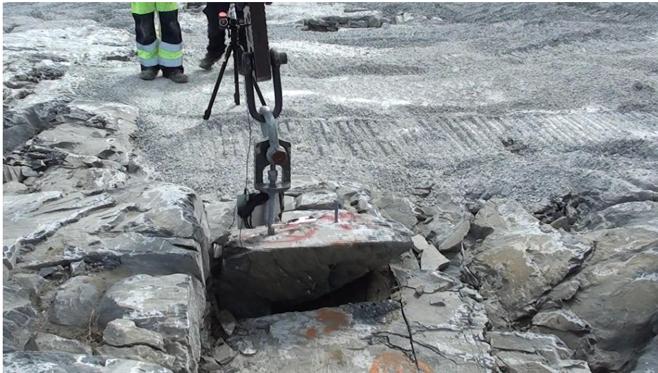
Figure 45 : Influence of structural geology on the shape of cone of rock mobilized by uplift anchors, Verdalskalk 2012, bolt nr 9
