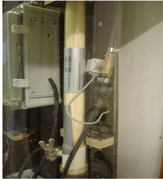
Figure 87. Membrane contactor used to provide bubble free aeration
