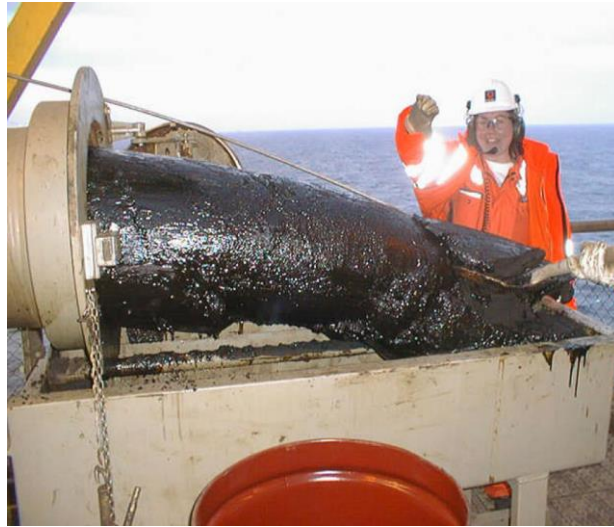
Figure 2-2 - A completely blocked pipe from the Norwegian shelf [13]
