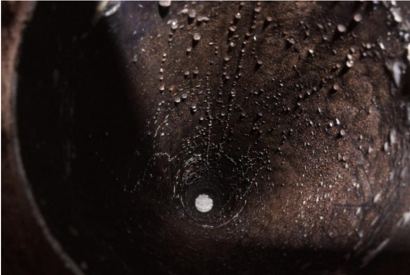
Figure 4-45 - Inside of pipe after wax removal. Test 2.2: Downstream coil movement, 15 kW output power.
