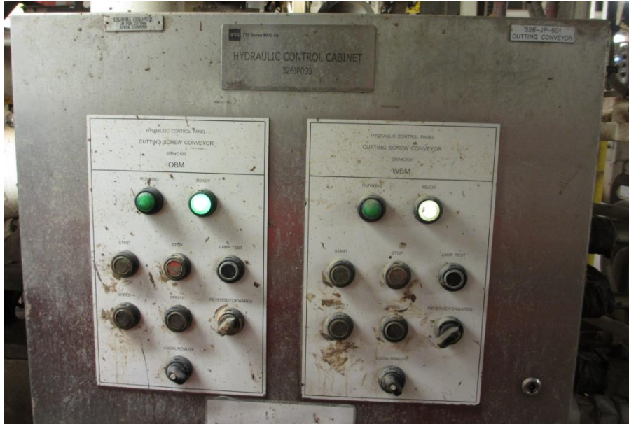
Figure 26 - Control panel for screw conveyors (photo: Sondre Buset Bjelland)
