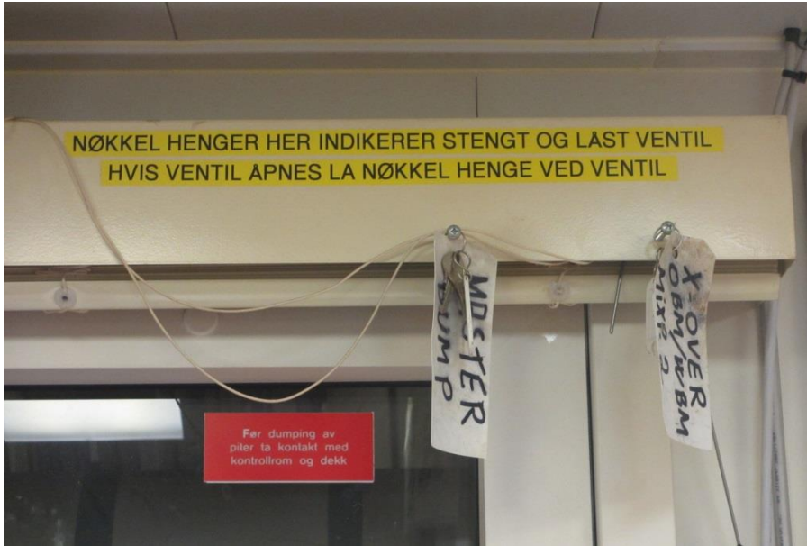
Figure 34 - Valve keys for valves without feedback (photo: Sondre Buset Bjelland)
