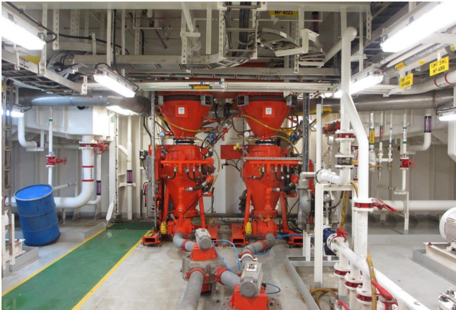
Figure 12 - The settling tanks with CRI (photo: Sondre Buset Bjelland)
