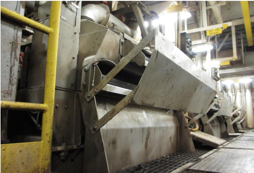
Figure 28 - Retrofitted shield in front of shaker (photo: Sondre Buset Bjelland)
