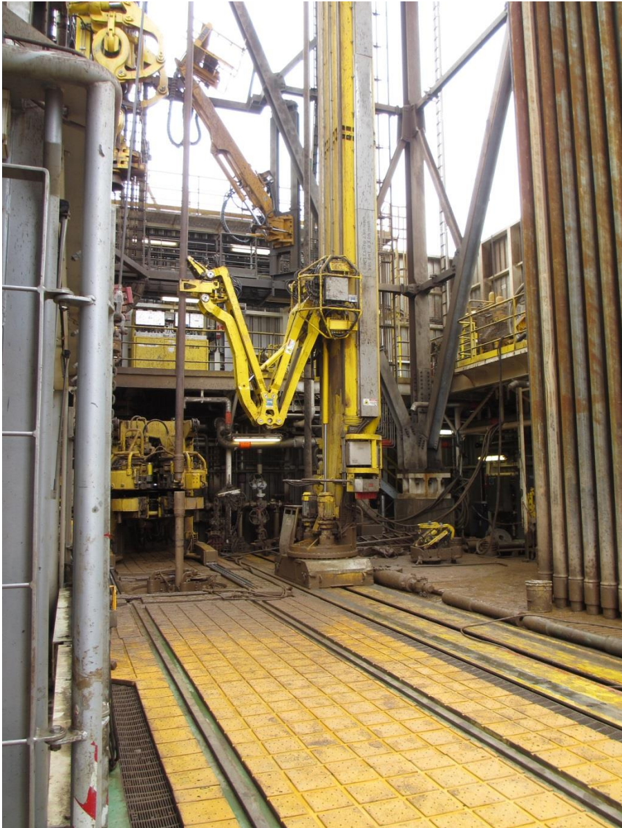
Figure 42 - Automatic pipe handling on drillfloor (photo: Sondre Buset Bjelland)
