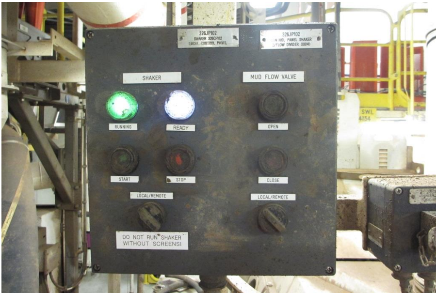
Figure 25 - Control panel for shakers (photo: Sondre Buset Bjelland)
