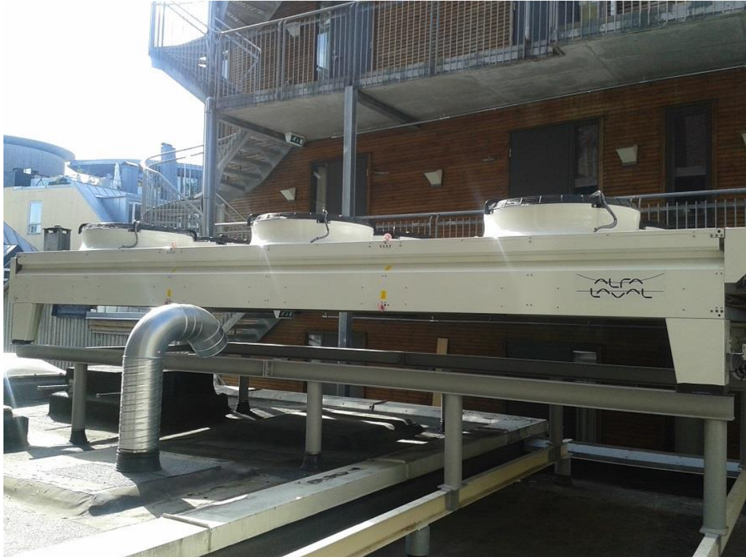
Figure 4.3 Gas cooler on the roof of Rema 1000 Prinsengata, side view
