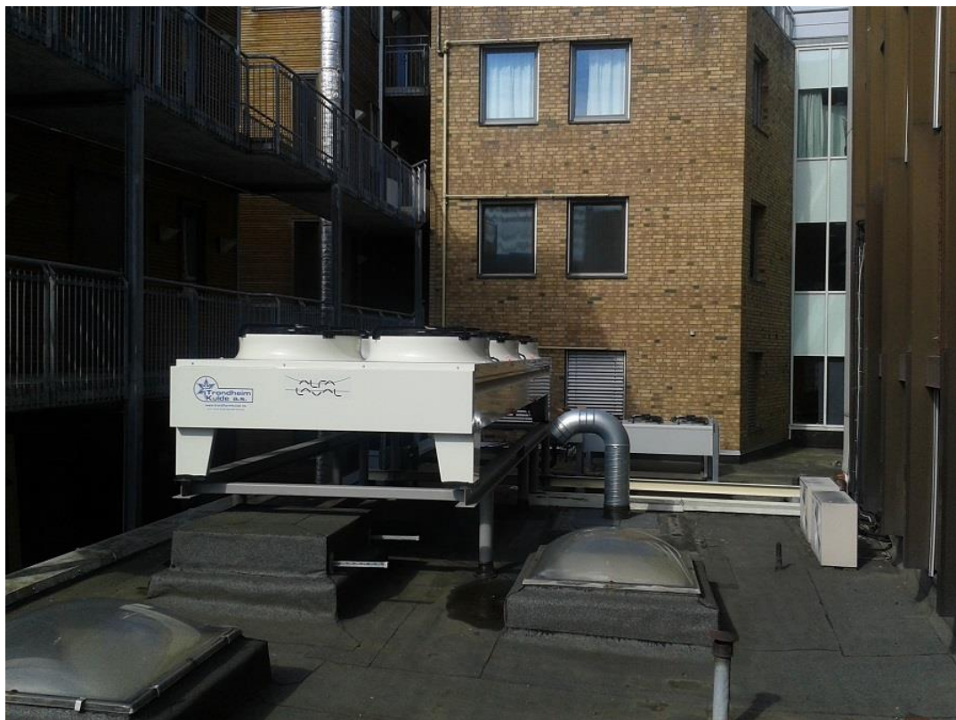
Figure 4.2 Gas cooler on the roof of Rema 1000 Prinsensgata, rear view
